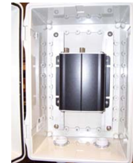
Photo #1 Encoder mounted inside enclosure
